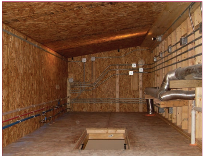
Photo 3: Electrical, plumbing and exhaust ventilation duct inside the conditioned attic space. Plumbing on the left side of photo are rainwater (white pipe), hot water (red) and city water (blue). Uninsulated exhaust air duct on right side of photo removes air from kitchen, bathrooms, and laundry room.
